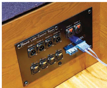
Madi optical cables connect the rooms
